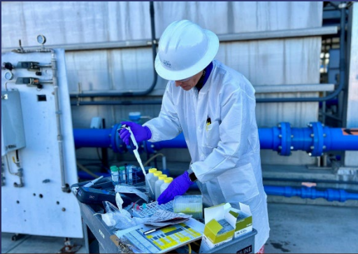
Performance Verification and Optimization with Monitoring
